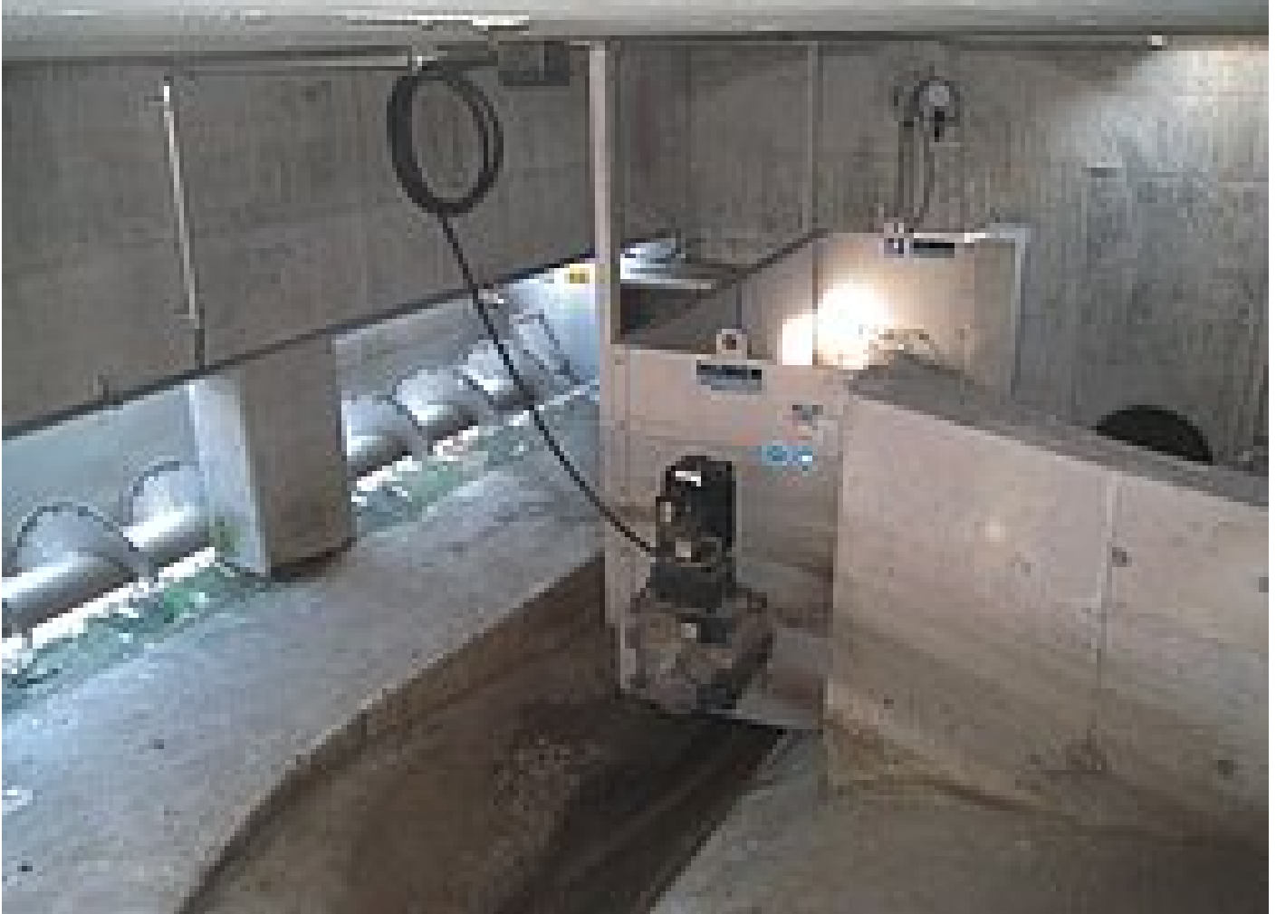
Stormwater overflow tank at Kappern: Storm Screen RoK1 on the left, Storm Screen RoK2 in the middle on top of the sewer towards the WWTP
