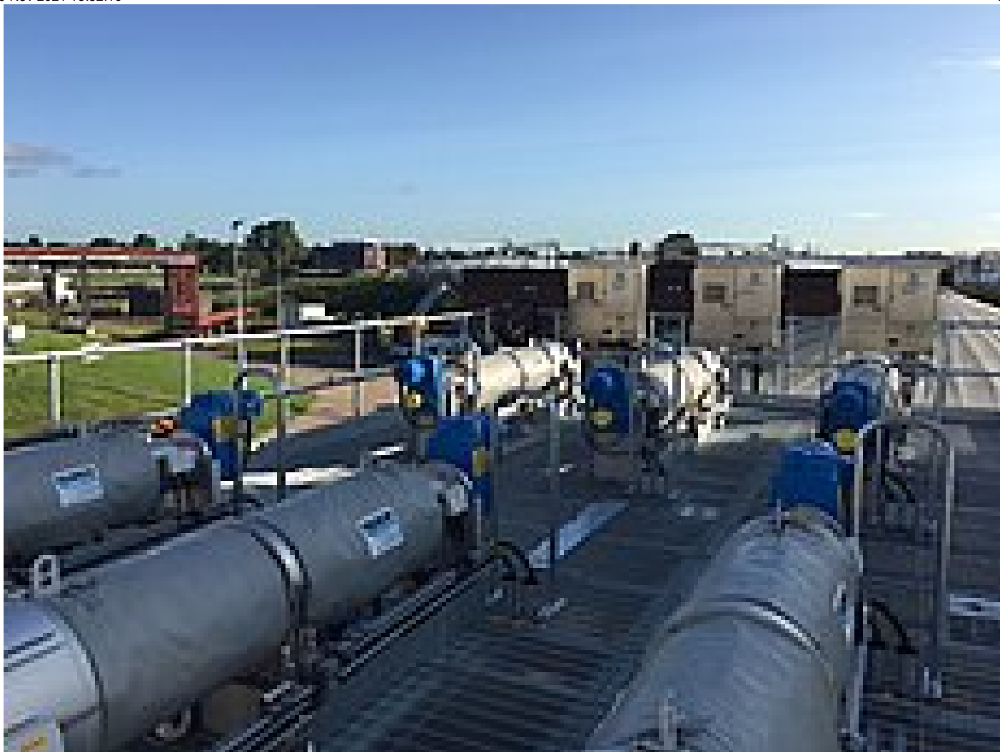
Minworth STW STRAINPRESS® Installation
