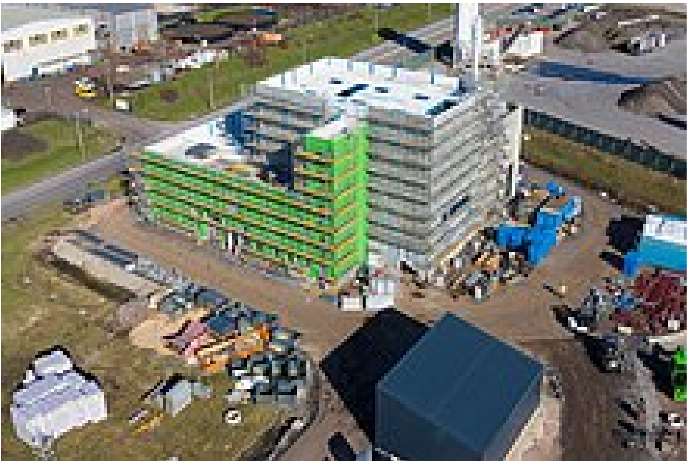
View of the sewage sludge incineration from above
