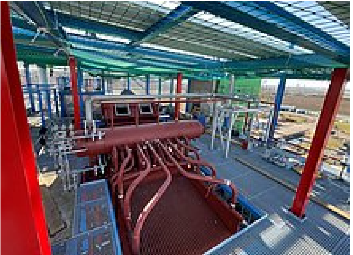
Steam drum of the sewage sludge incineration plant
