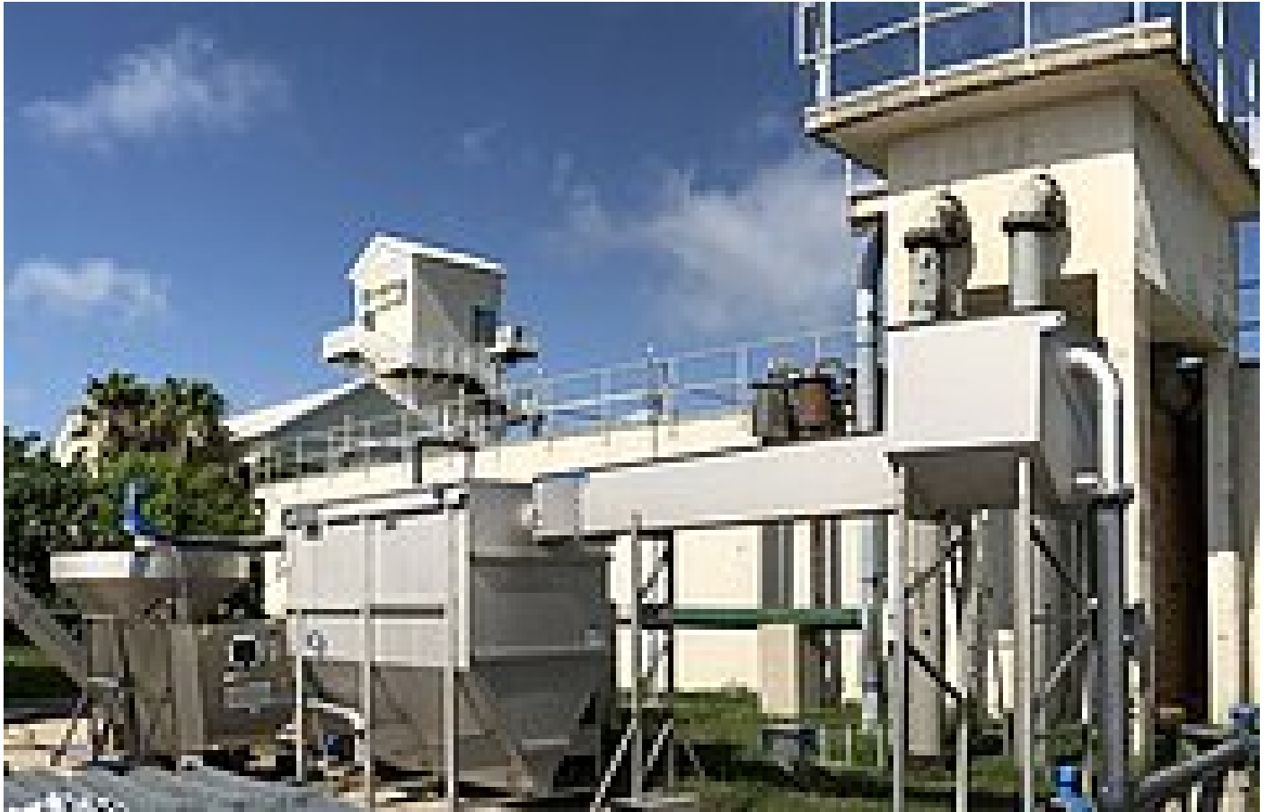
Test stand to determine the separation efficiency of the HUBER Grit Trap GritWolf® at 40 °C in South Padre Island, TX
