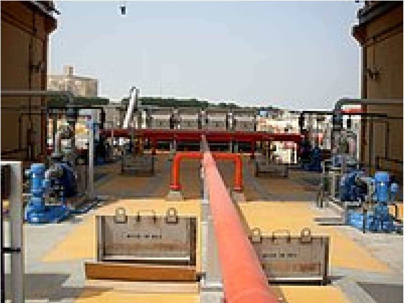
Installation with a set of 4 VORMAX units
