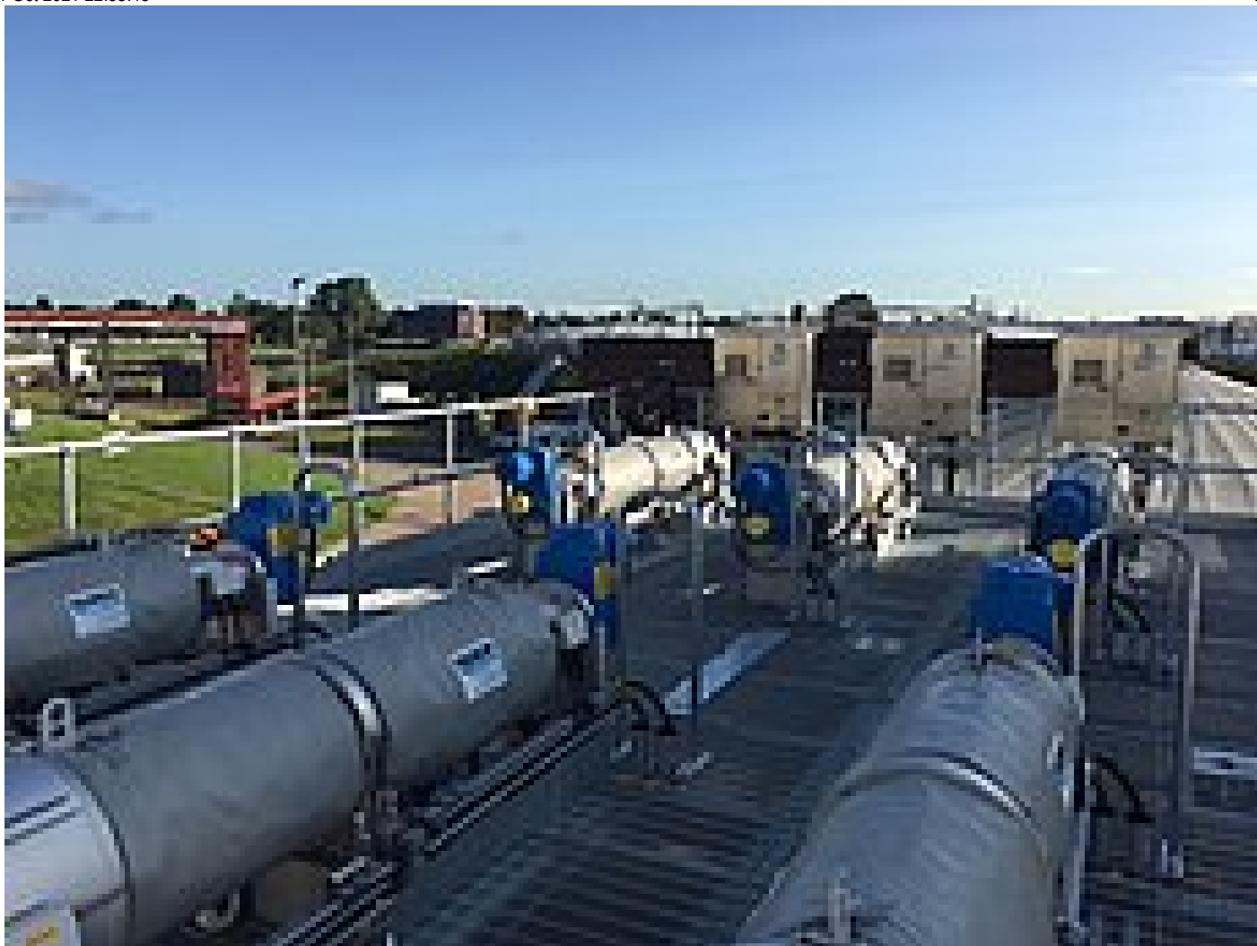
Minworth STW STRAINPRESS® Installation
