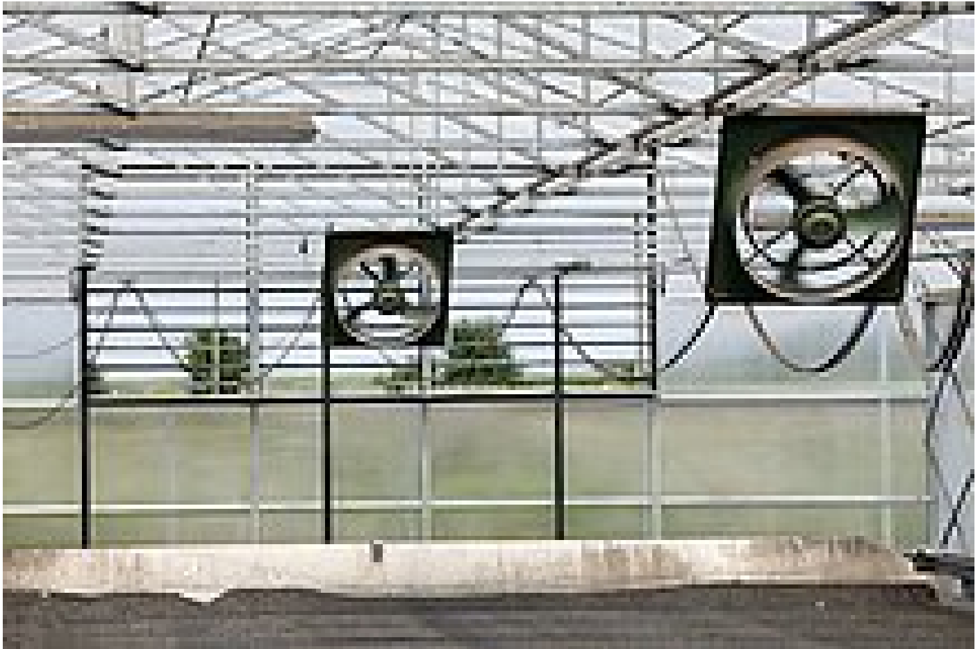
At the end of the drying surface a light stainless steel construction is used. Roads, turning round areas or big gates are not necessary.
