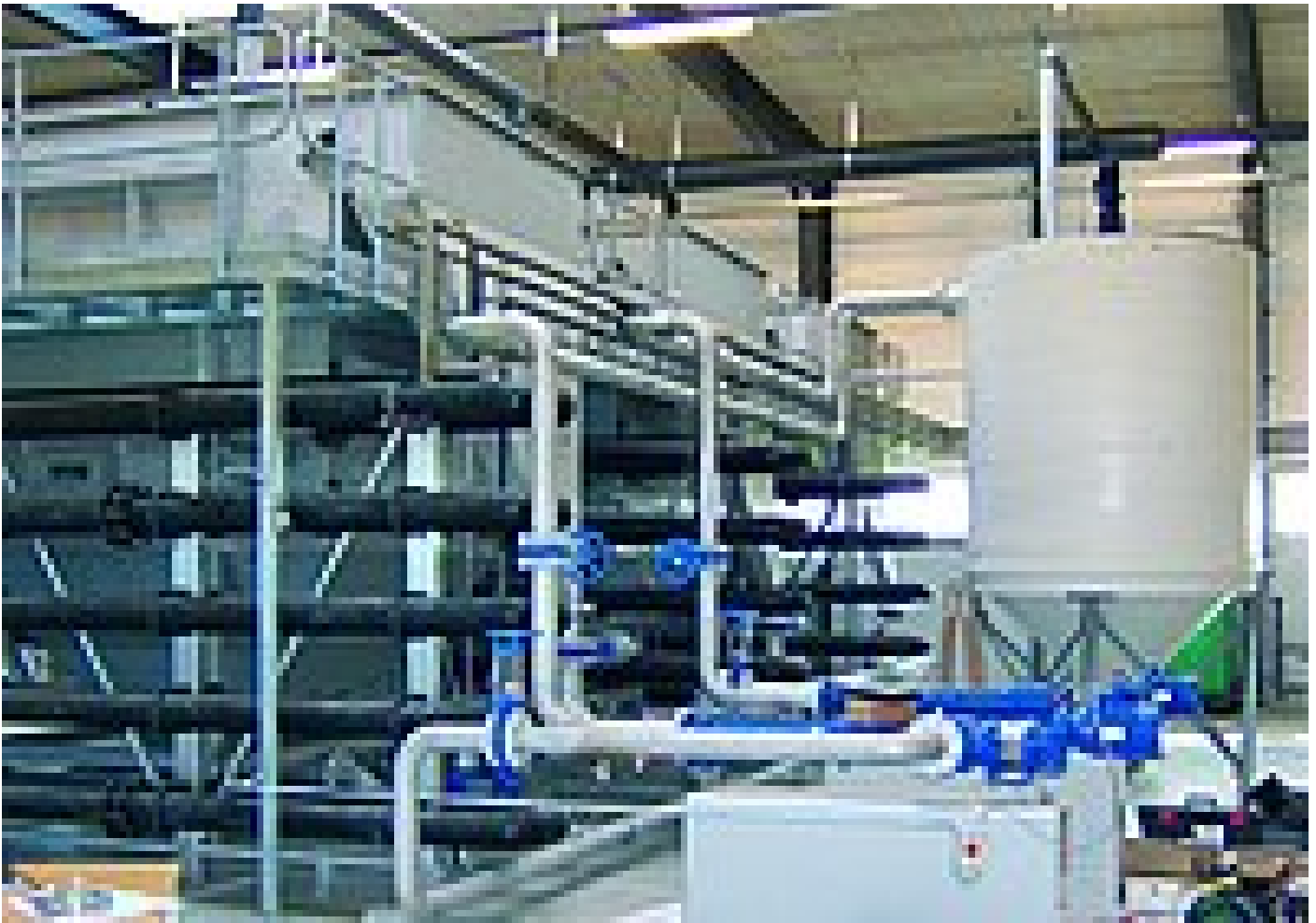
Three HUBER dissolved air flotation units HDF-7 with tubular reactors for chemical pre-treatment and sludge storage tank
