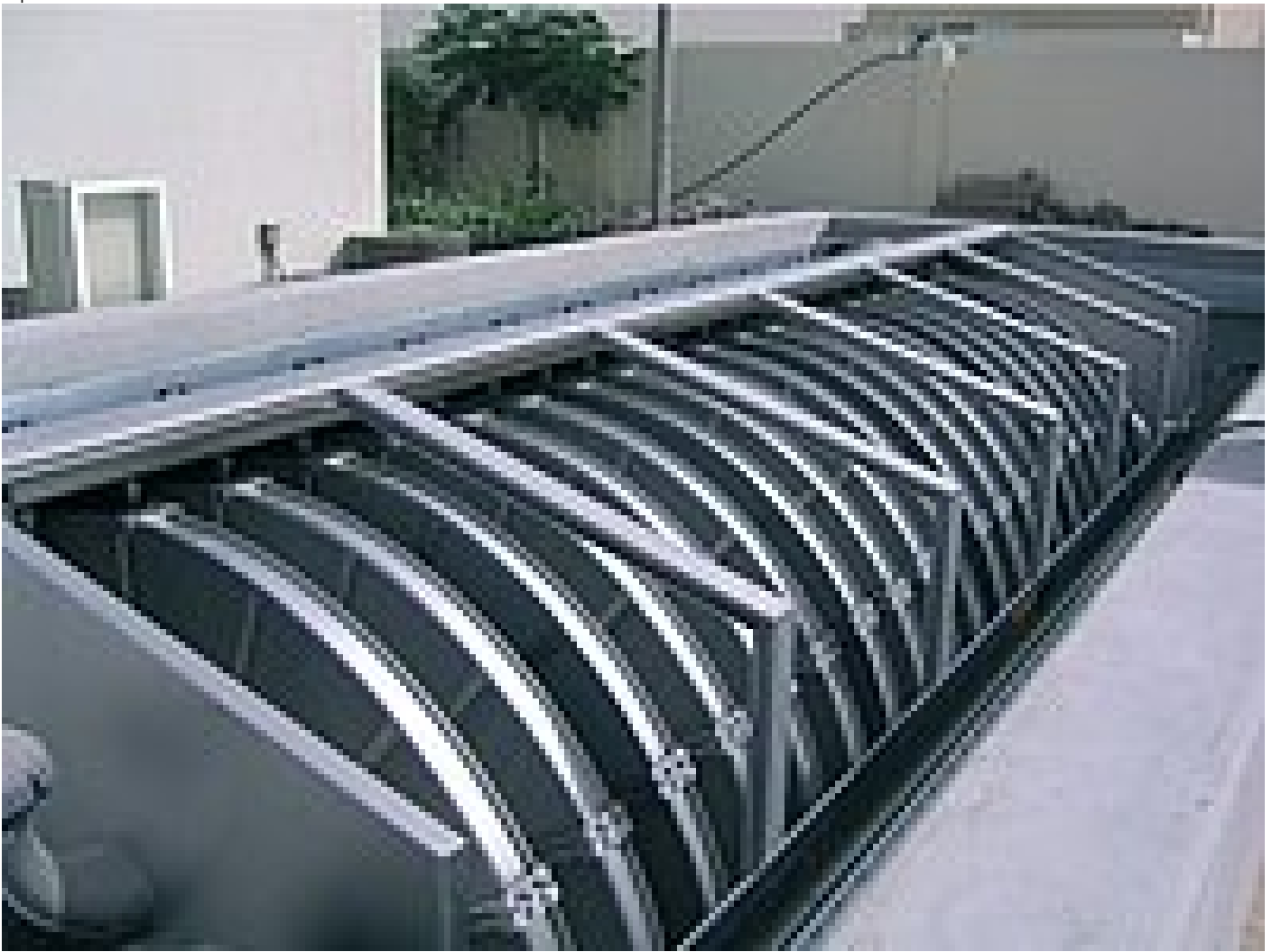
RoDisc® 20 in concrete tank at the Al Sweihat pumping station in Sharjah, UAE
