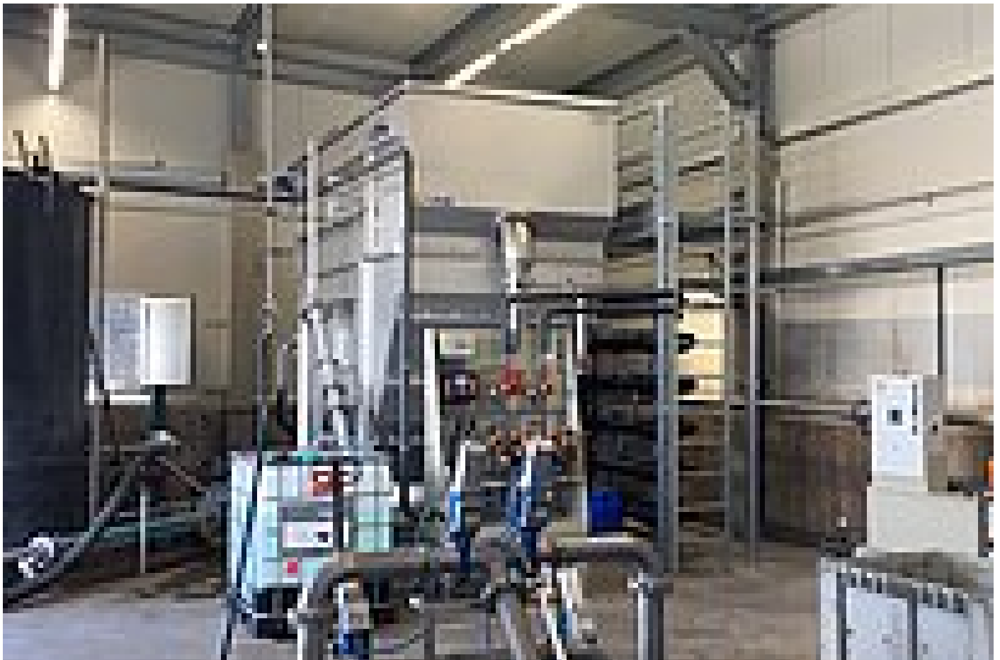
HUBER Dissolved Air Flotation Plant HDF10 with chemical treatment stage
