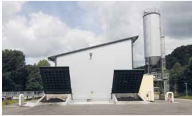
Sludge bunker and dry material silo.
