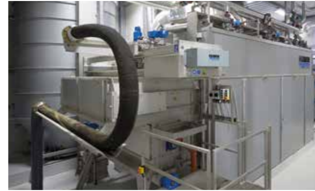
Sludge feeding with HUBER extruder unit (pelletizer).
