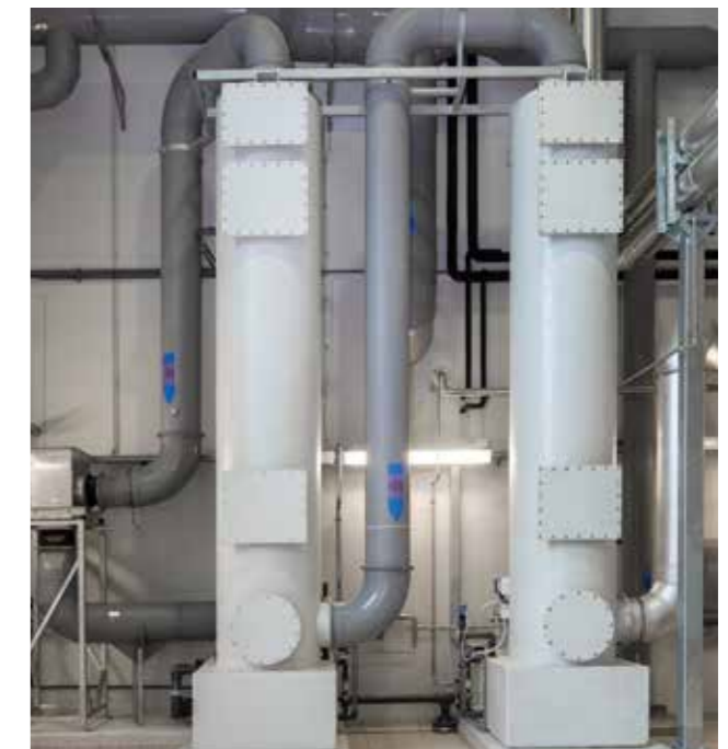
Two stage scrubber for odor control.
