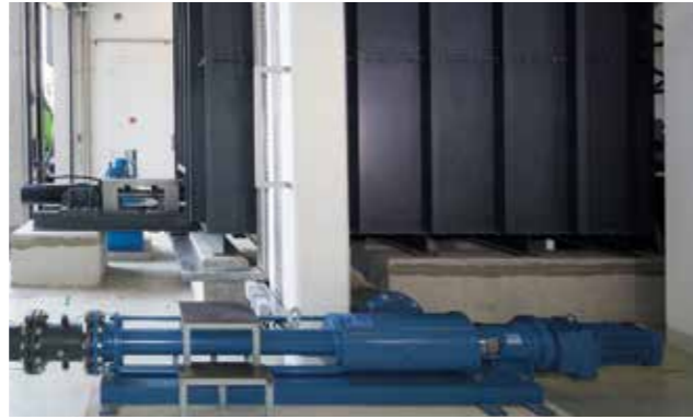
Sludge bunker and pump.
